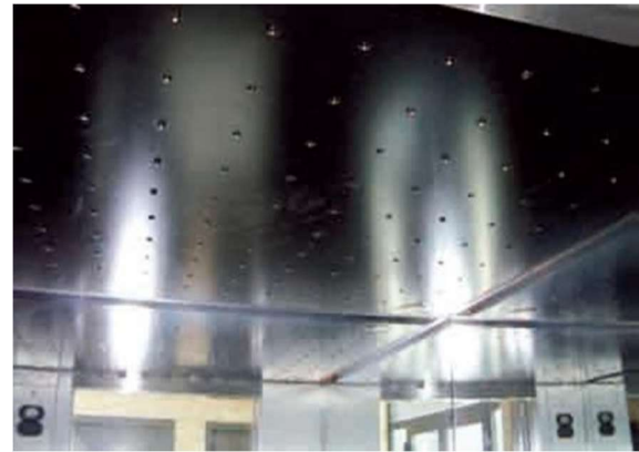
Figure 8 - Elevator car ceiling illuminated with individual LEDs.
